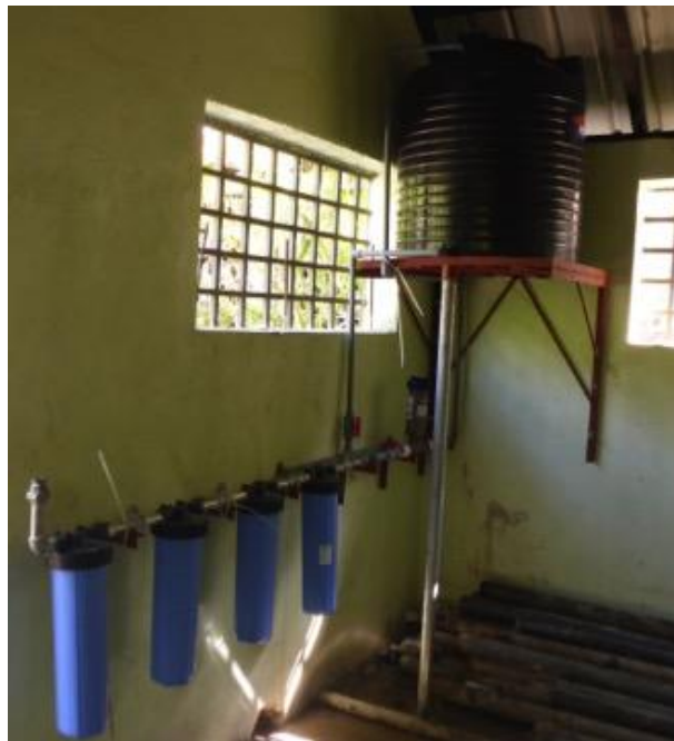
FIGURE 5 COMPLETED BA CANGE WATER TREATMENT SYSTEM.
